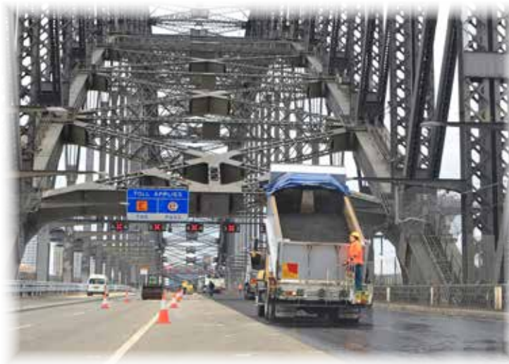
SAMlseal S45R on Sydney Harbour Bridge
