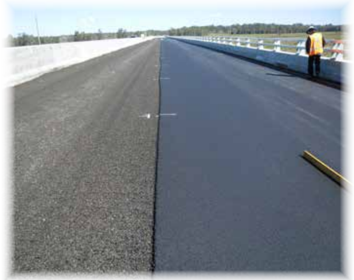
SAMlseal S25E, SAMlseal S20E on Australia's Longest Bridge - Macleay River and Floodplain Bridge, Pacific Highway
